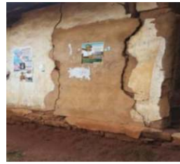
Figure 1: Building abandoned at Mbiama because to cracks
