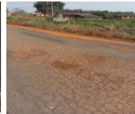
Figure 2: Failed portion of road at Mbiama
