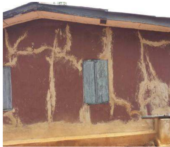
Figure 3: Patched cracks on the wall due to Expansive soil at Mbiama
